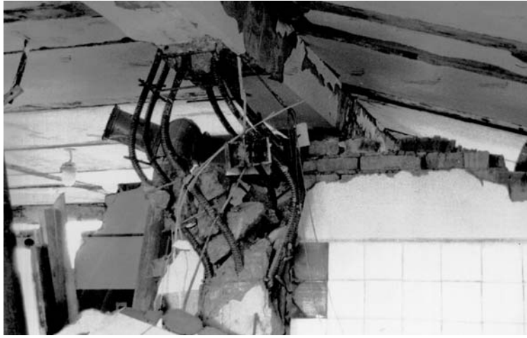
Fig. 1. Failure of the middle reinforced concrete column of the ground floor of the service center building at the Goryachie Klyuchi village (the Iturup island) as a result of an earthquake of magnitude 7.9.
